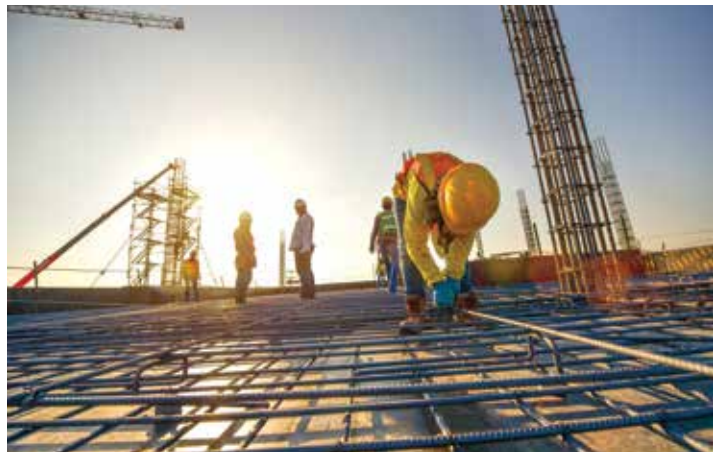
▲ Construction of steel buildings requires well-planned placement of steel fittings and attachments.
