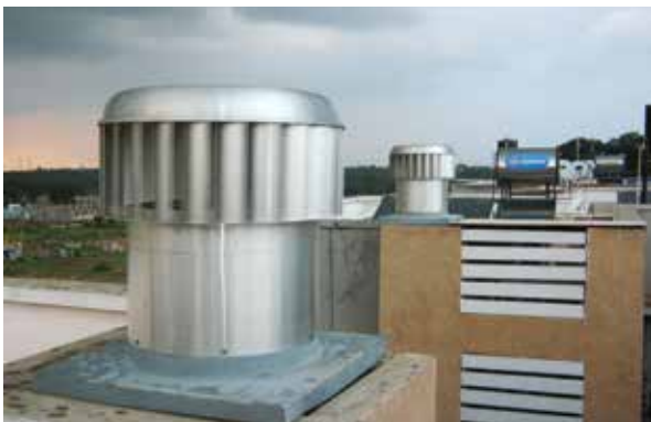
▲ Ventilation systems take up plenty of space place in terms of coolers and blowers.
