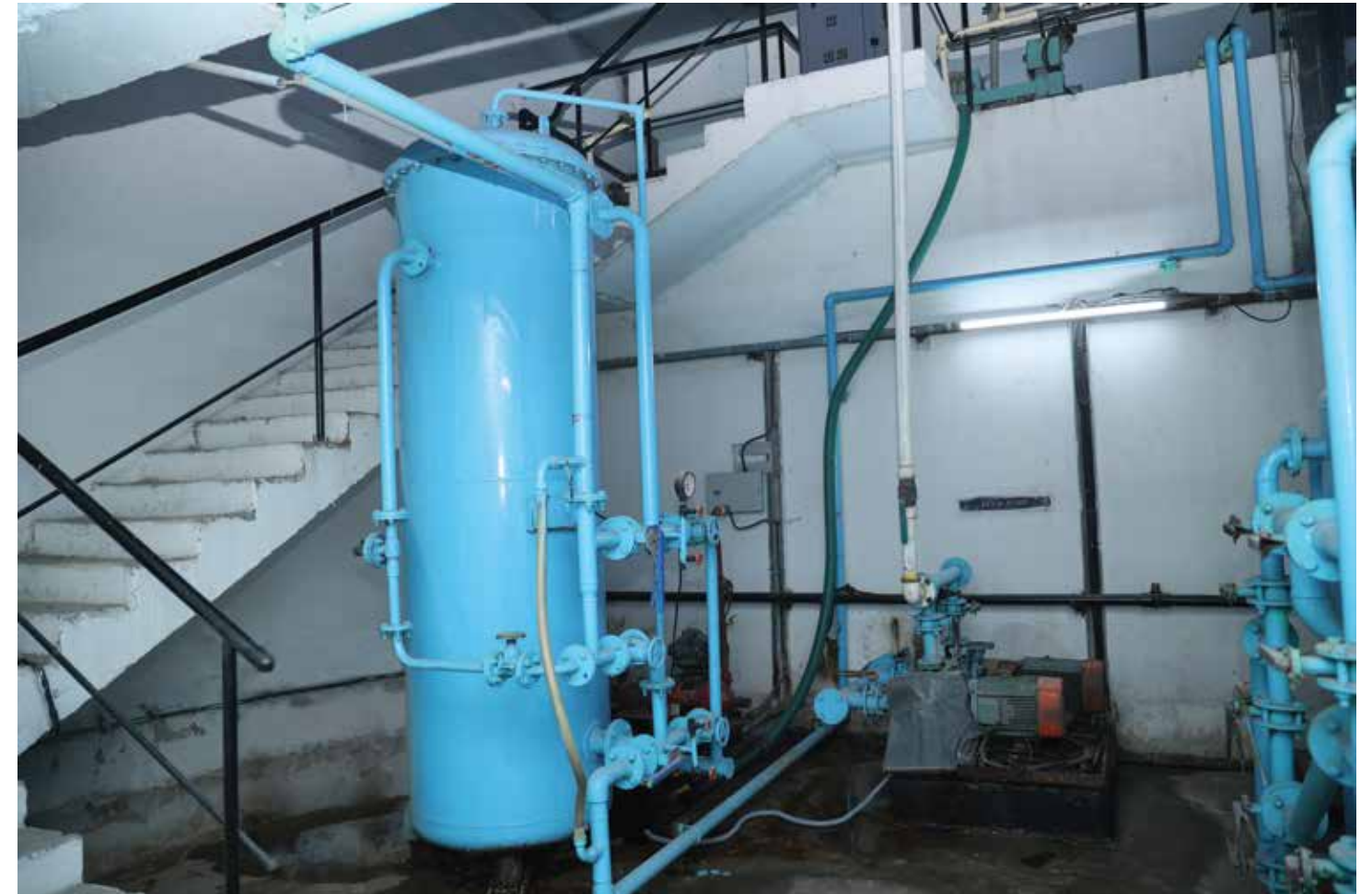
➔ Water filtration system at Sheraton Hyderabad.
