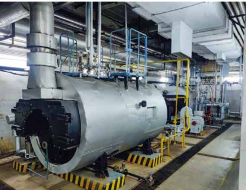
Educational tours to showcase eco-friendly practices (boiler plant) at Le Meridien Gurgaon, Delhi NCR
