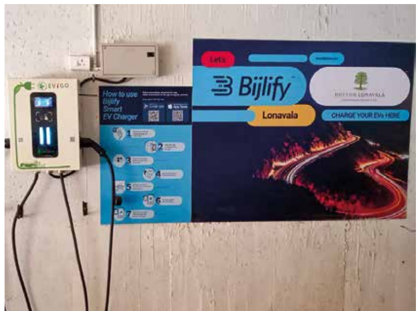
EV charging station at Rhythm Hospitality
