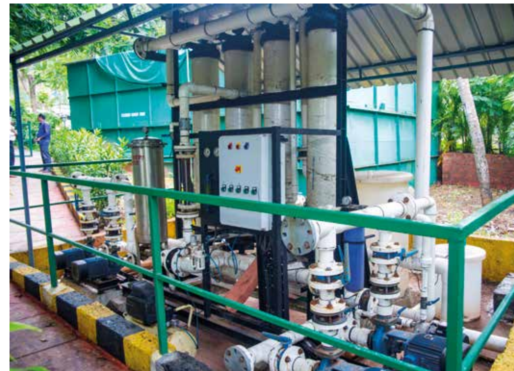
Sewerage treatment plant at Fort Aguada
