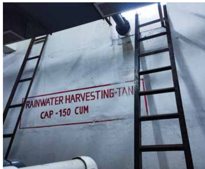
Rain water harvest tank at JW Marriott Mumbai Sahar
