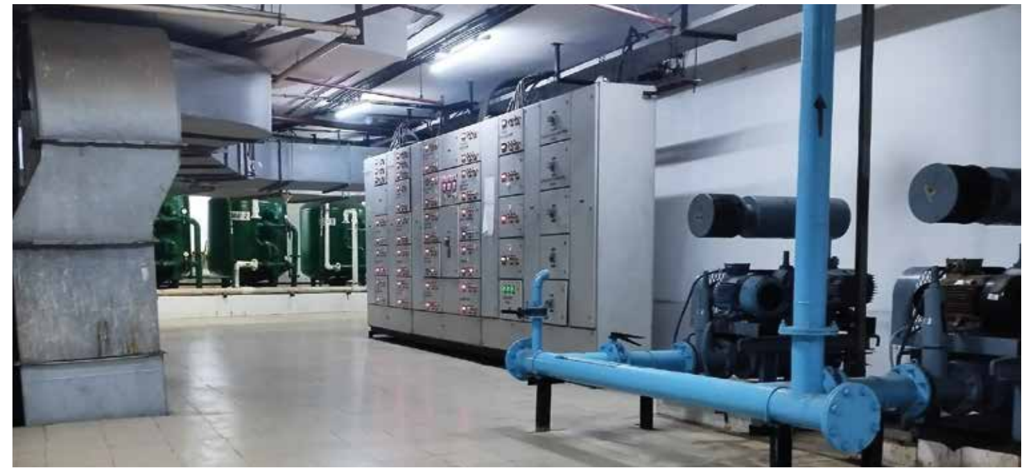
Sewage treatment plant (STP) at JW Marriott Mumbai Sahar
